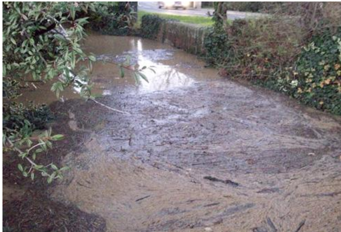
The junction of the small watercourse around Greatford Gardens with the drainage ditch alongside Carlby Road. The water is backing up against the brick front of the overloaded culvert under Carlby Rd (constructed 1837). The water height is above the flooded arch. Christmas 2020
